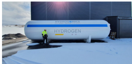
The hydrogen tank outside the containment building
