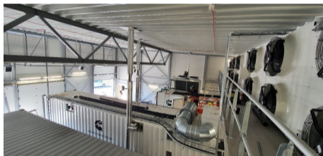
The electrolyser & rectifier containers within the containment building
