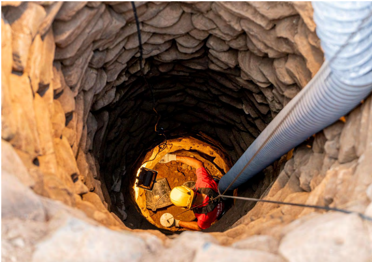
Figure 23. The technician digging a dry well. Image courtesy of Archéologie des Puits.
