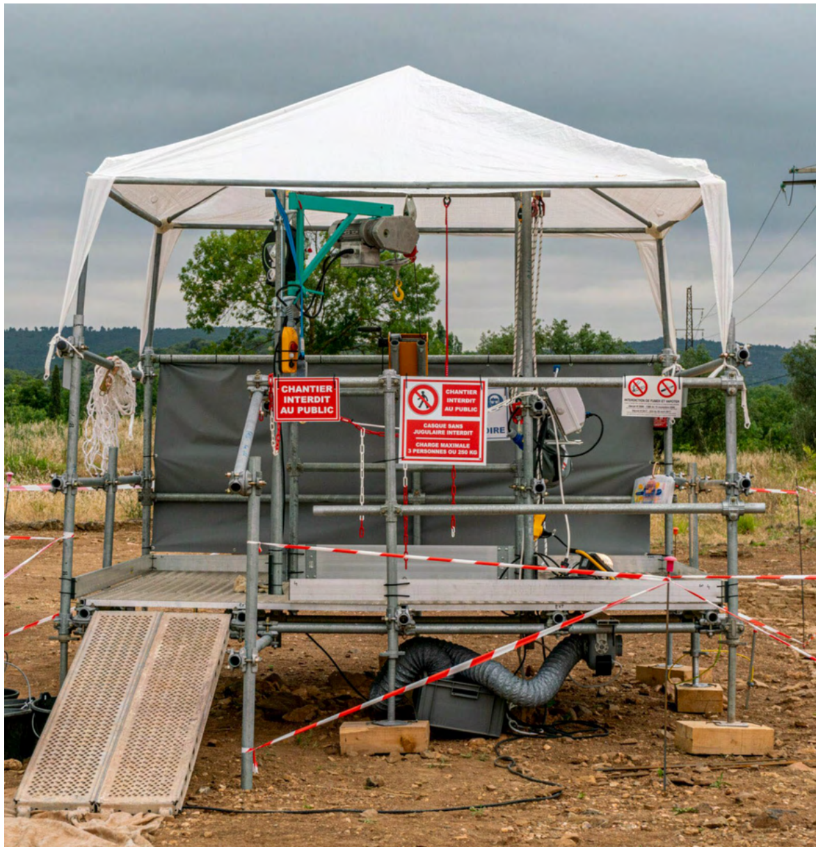
Figure 21. ADP’s platform equipped and ready for the dig. Image courtesy of Archéologie des Puits.
