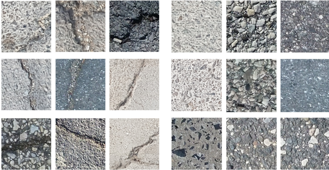
Figure 2. Samples of crack and non-crack patches.
