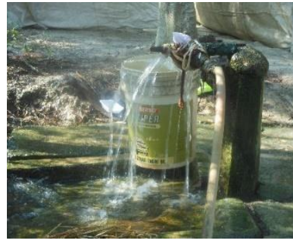
Plate 6: Pipe Line Water Of Amaravati Village Of Namkhana Block
