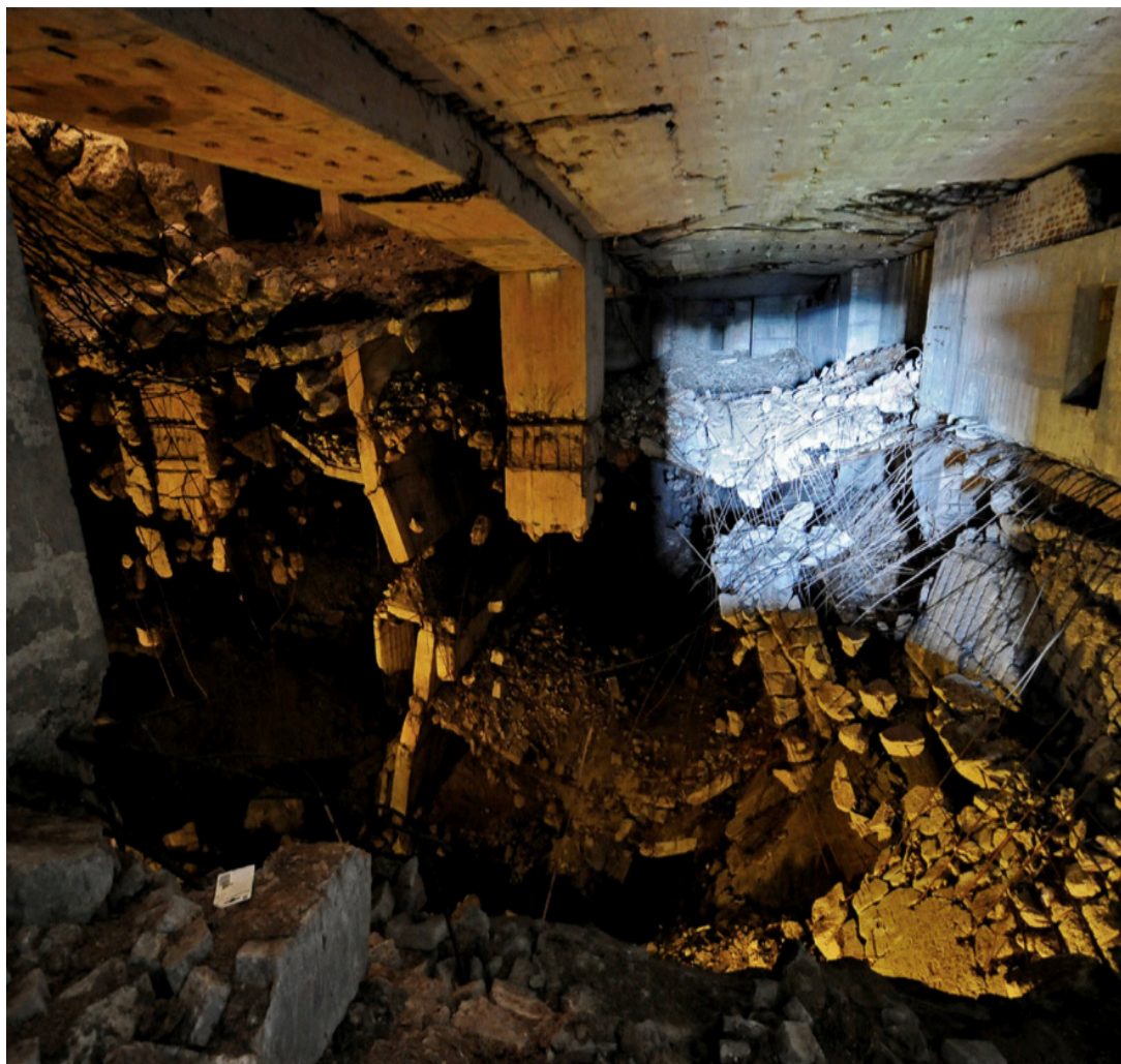
Fig. 9: The damage inside the Bunker
