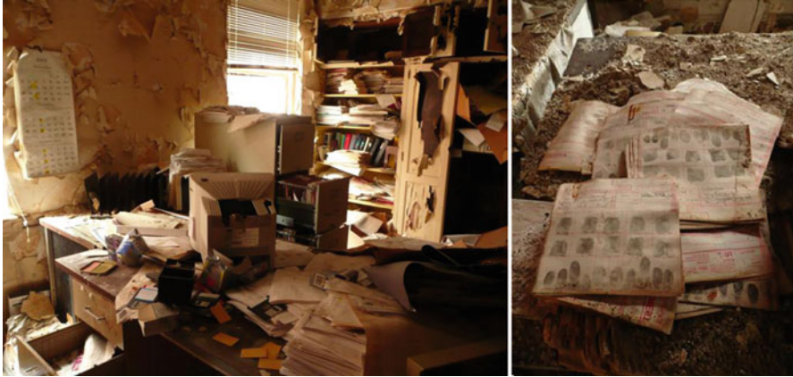
Fig. 9.2 Pictures of an abandoned police station in the Detroit Area (USA), showing fingerprints and other personal data scattered on the floor
