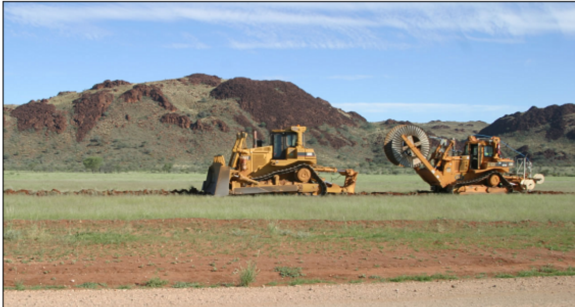
Figure 4 - The fibre optic cable being laid near Blackstone community. (Photo: Daniel Featherstone/ Ngaanyatjarra Media)
