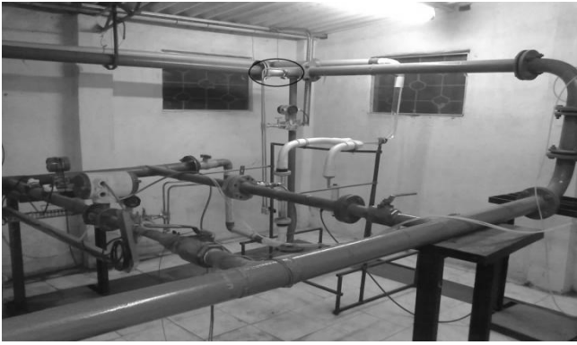
Fig.A2. Experimental setup with leak position 3 near elbow (encircled)
