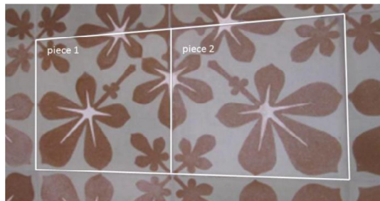
Figure. Hydraulic mosaic tiles, piece 1 without discoloration and piece 2 with discoloration.
