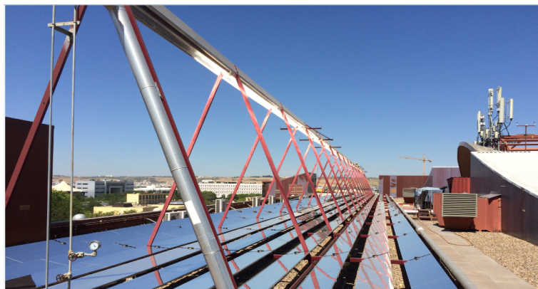
Figure 2. Fresnel collector field.
