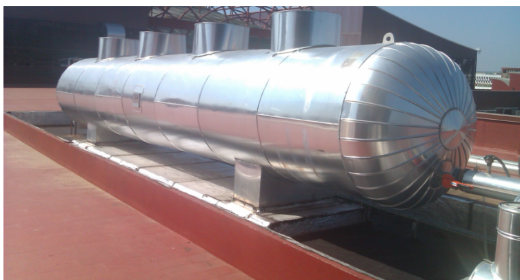
Figure 3. PCM storage tank.
