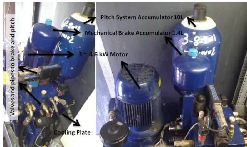
Figure 7. Hydraulic unit of pitching system (Turbine VESTAS V39/V4x/V90). [24] [24]
