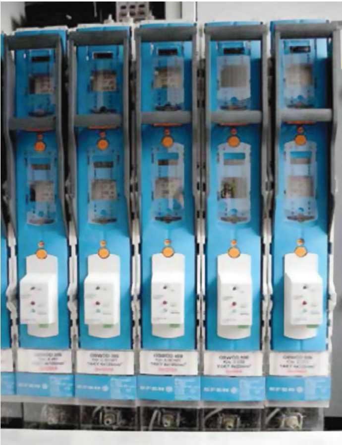
Fig. 3. Example of LV switchgear with fuse blow-out indicators, a blow-out signal is forwarded directly by SCADA to the grid operators
