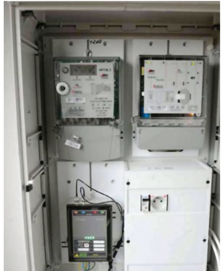
Fig. 1. Cabinet with balancing system installed in an MV/LV transformer substation building
