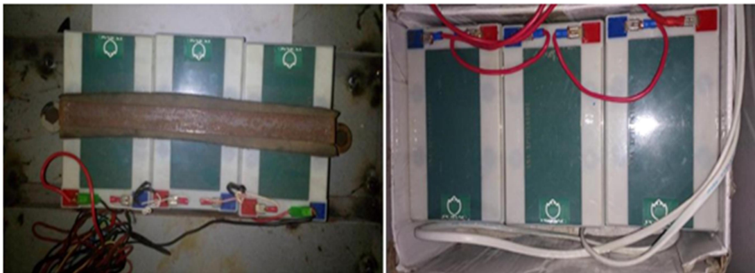
Fig 2.5: Two sets of batteries
